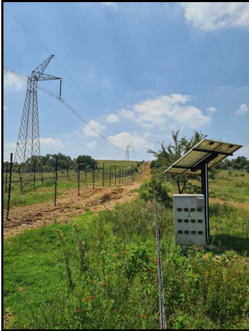
Figure 3: The 2.4-meter game proof electric fence with solar back-up around the property
